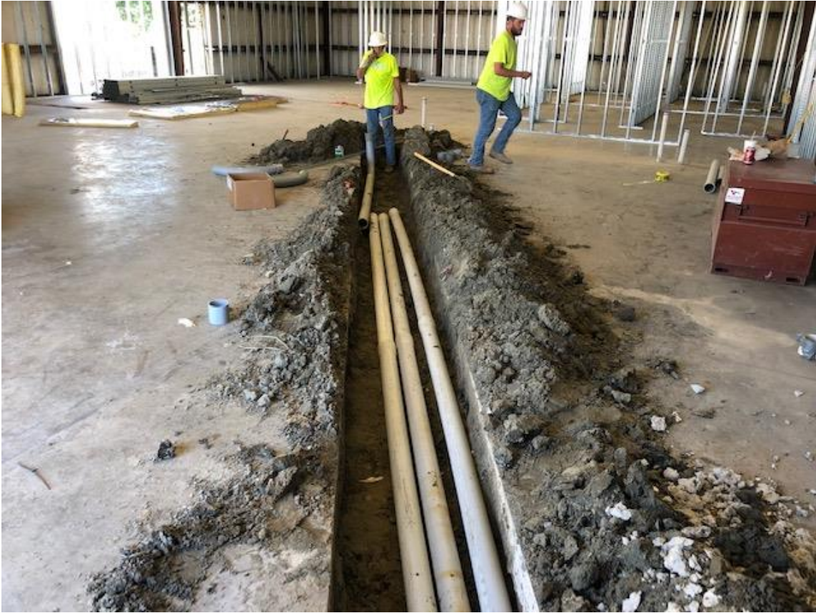
The electrician is roughing in the electrical chase ways for the power upgrade.
